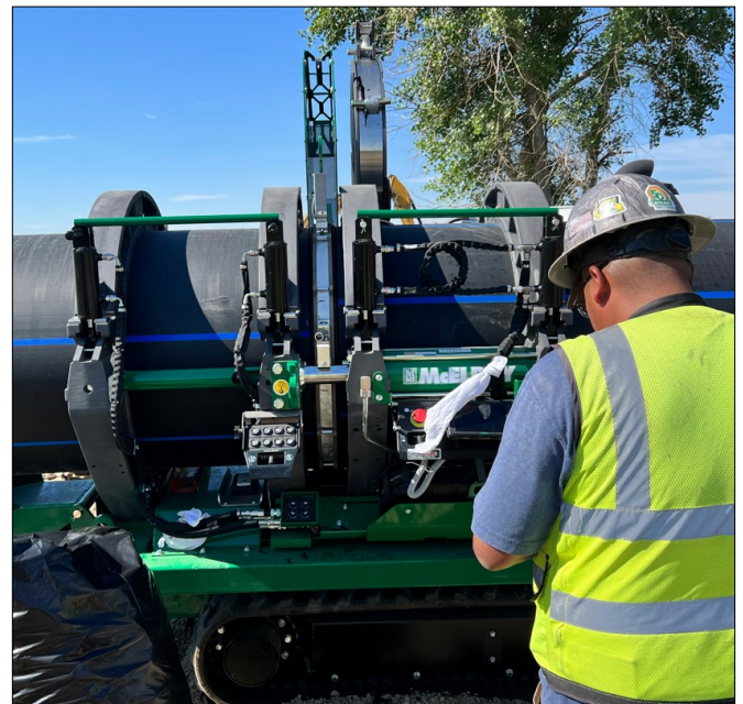
30-inch HDPE pipe is welded by a WCA employee along Boone Reach 1 as part of the AVC Reclamation Sub-Project.
